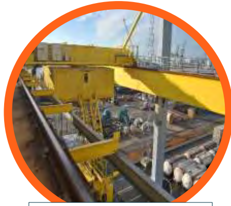
Cranes Trolley Tracks
