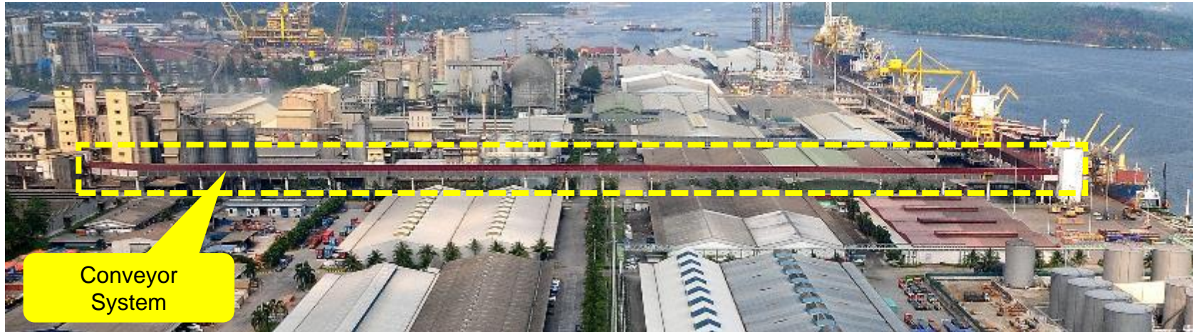
Installation of new Conveyor Belt for Cereal Conveyor System at W4, W5, W6 & W7 & connected to LL1, LL2, LL3 and BG1.
