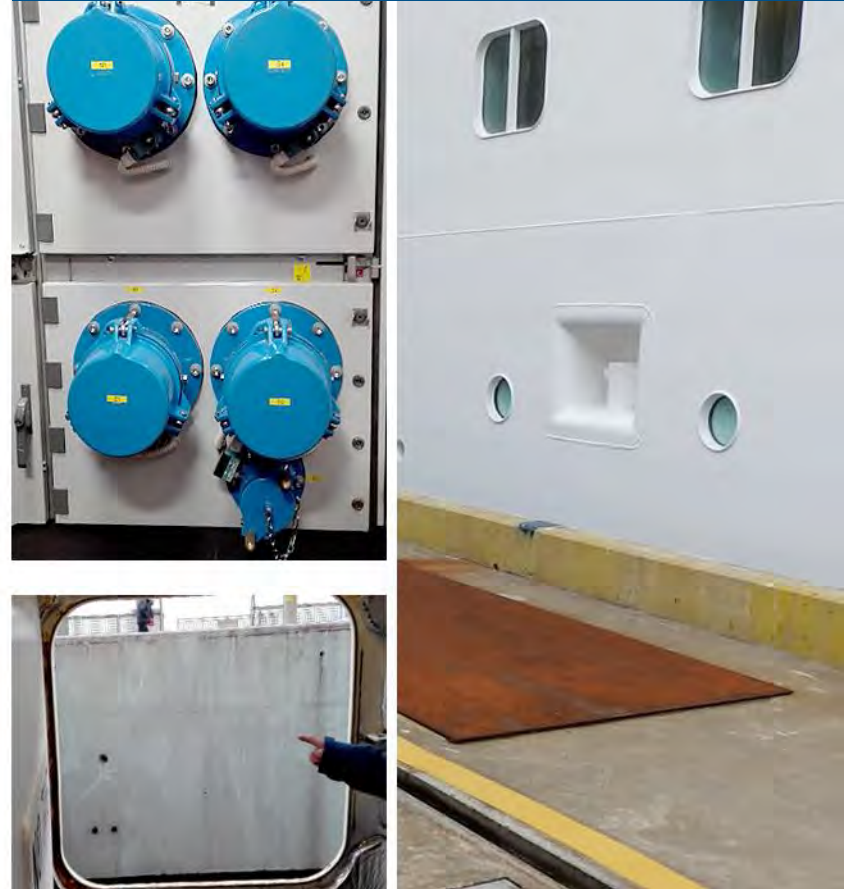
Ship's hatch / Control Cabinet
