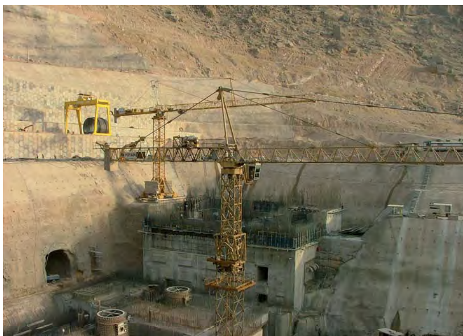
Dam– Gantry Crane 40/5 Ton with 50 meters lifting height for installation of the pipes of dam.
