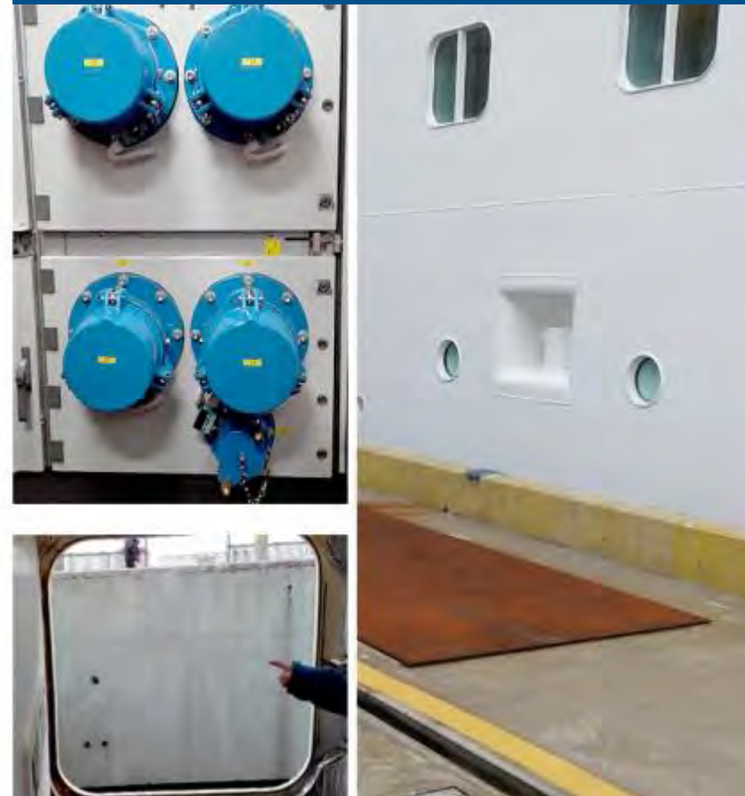
Ship's hatch / Control Cabinet
