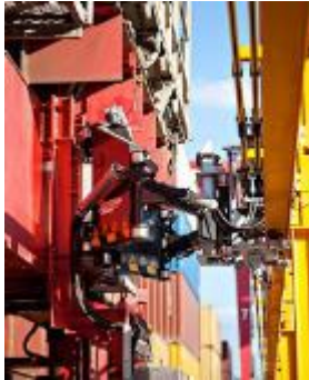
Yilport, Turkey Electrification of 18 non-Kalmar RTGs ▪ Installation and commissioning of pneumatic actuated automatic drive-in units ▪ Conductor bar system
