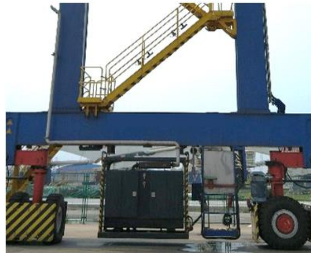
Small diesel genset mounted under sill beam
