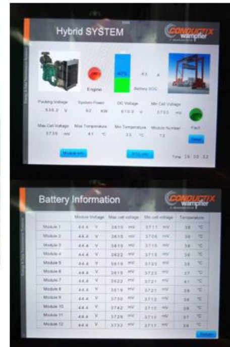
HMI Touch Panel
