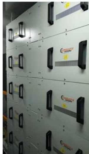
Battery modules inside the housing
