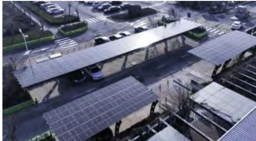
Photovoltaic clean energy
