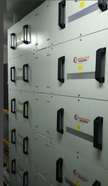
Battery modules inside the housing
