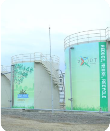
Oily Waste Water Treatment Plant
