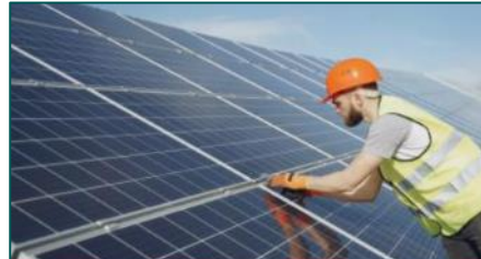
Solar collectors have been installed on the roofs of the Freeport of Riga buildings
