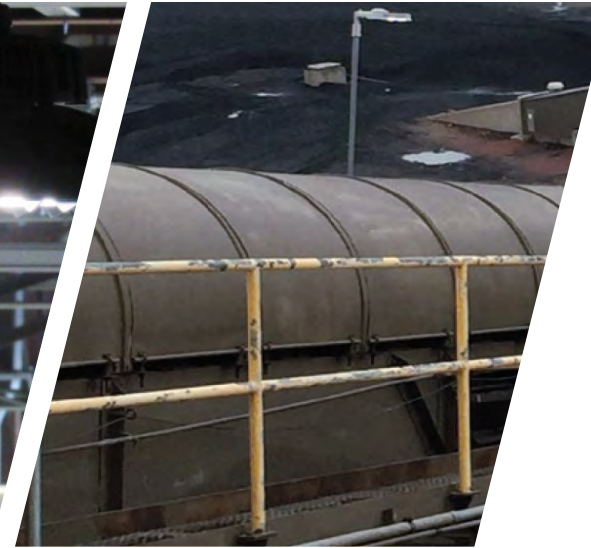
CONVEYOR BELT SYSTEMS
