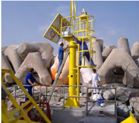
SERVICE, INSTALLATION AND MAINTENANCE
