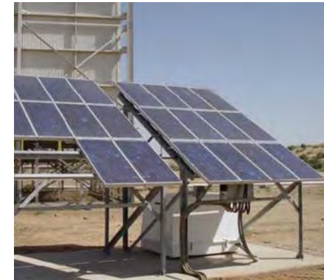
SOLAR POWER SYSTEMS
