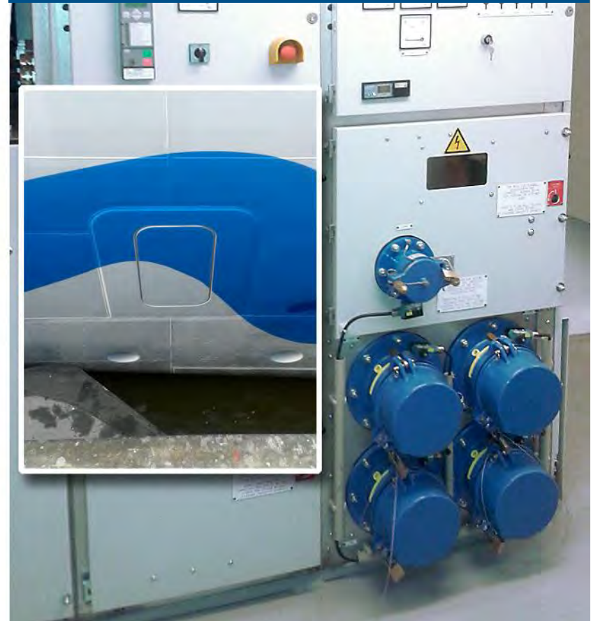
Ship's hatch / Control Cabinet
