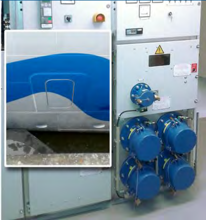
Ship's hatch / Control Cabinet
