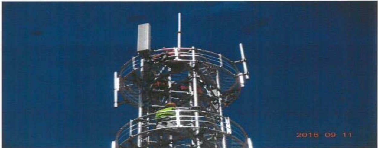
P10: Feeder of Base station No.21 of Section 11 (11 Sep, 2016 DK234)
