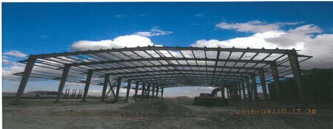
P8: Structural Steel of Rolling Stock Depot of Section 8 (10 Sep 2016 Nairobi South)
