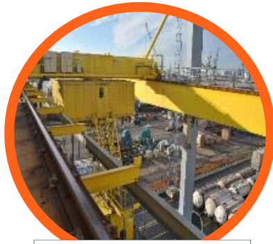
Cranes Trolley Tracks
