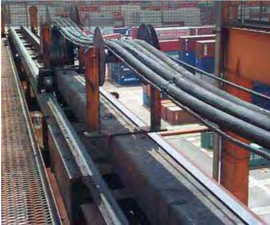
Before: Cable tender
