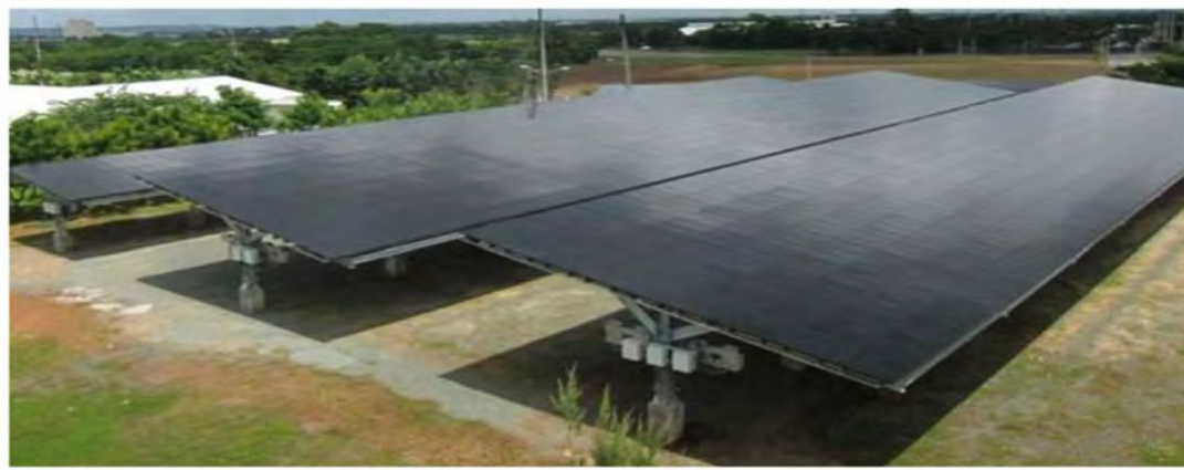
206.5 kWp Solar Carpark & Test Bed Canlubang, Laguna, Philippines
