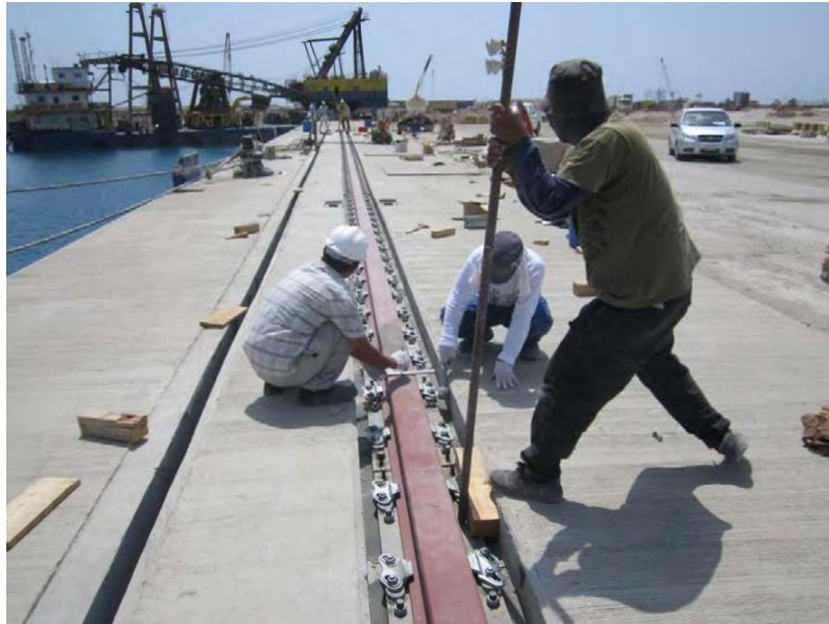
STS track installation in KAEC Port, Saudi Arabia (A150 rails, RailLok W25 clips, 35m span)
