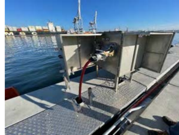
10 kV distribution box
