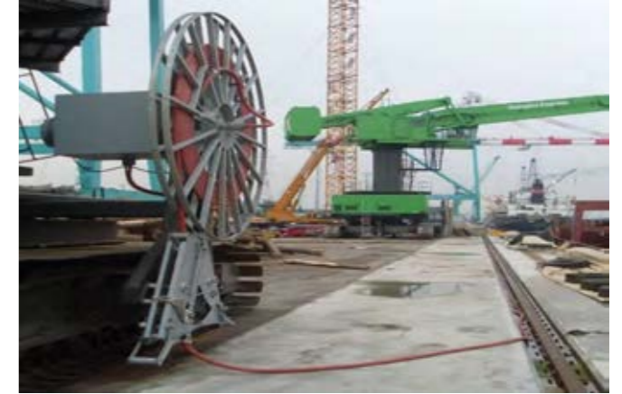
Open cable channel
