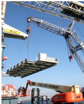
Rotterdam, the Netherlands Upgrade of 12 non-Kalmar STS cranes ▪ 8-metre height increase ▪ 4-metre boom extension ▪ Stacker platform ▪ Lifetime extension
