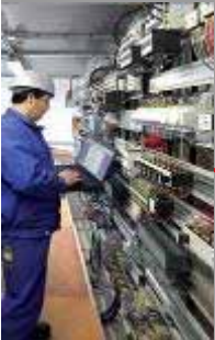
Generously sized electrics room
