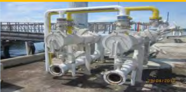
The manifolds on the loading platform
