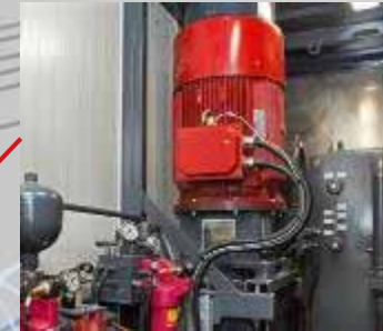
Hydraulics room with main pump and tank
