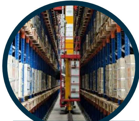
Automated Storage and Retrieval System
