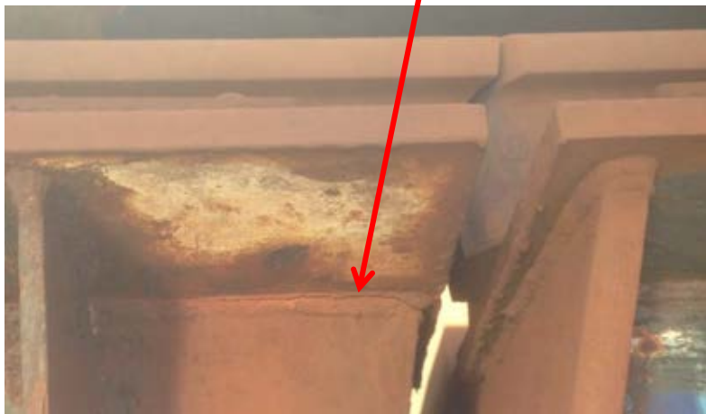
Stringer Structural Fatigue Cracks
