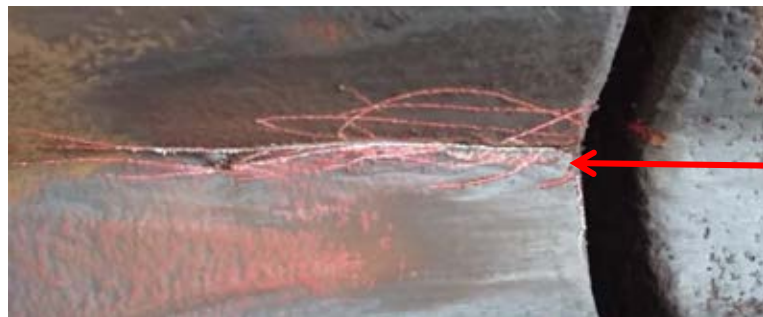
Potential Structural Crack
