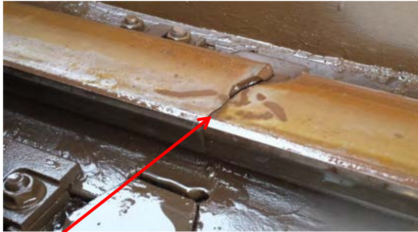
Rail and weld cracks
