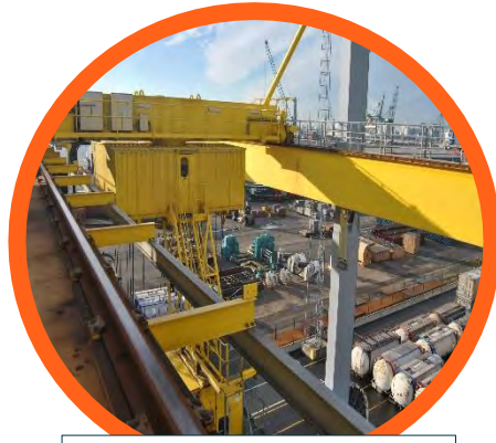
Cranes Trolley Tracks
