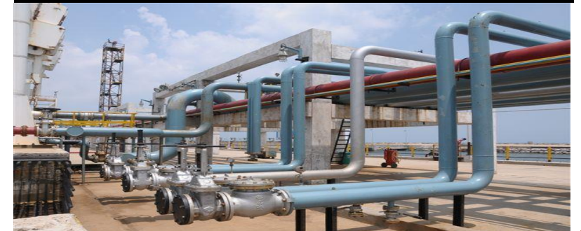
Typical Pipelines on jetty (planned)
