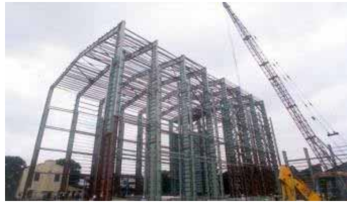
Garden reach ship builders & engineers limited - Modernisation of hull shop – II (phase I)
